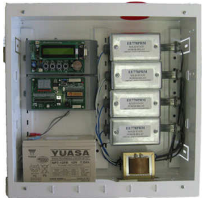
eBox set-up with eTimer and 4 ePower Relays (for high voltage application)
