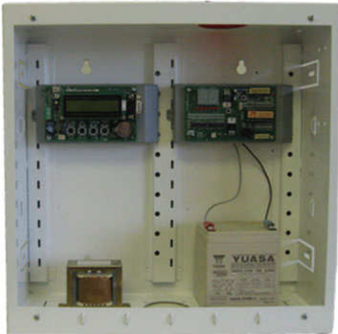
eBox set-up with eTimer (for low voltage application)
